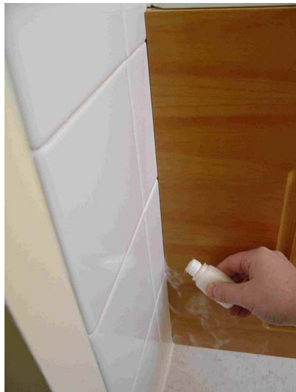
Figure 15 - Leak around Bath Panel (Plot 16)
