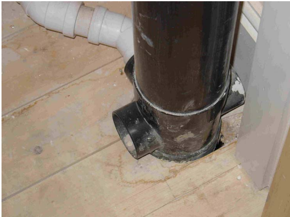
Figure 21 - Gap around Soil Vent Pipe in Floor of Boiler Cupboard (Plot 17)
