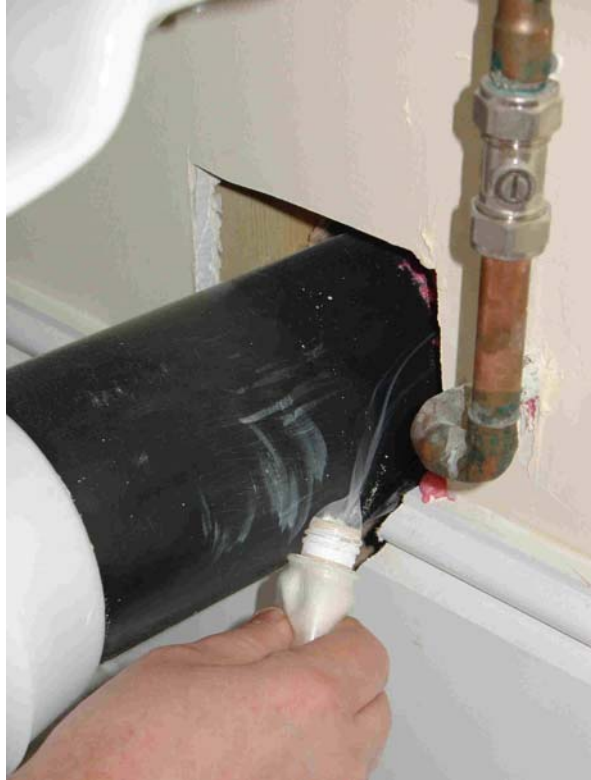
Figure 14 - Leak around Soil Pipe Penetration in Downstairs Toilet (Plot 17)
