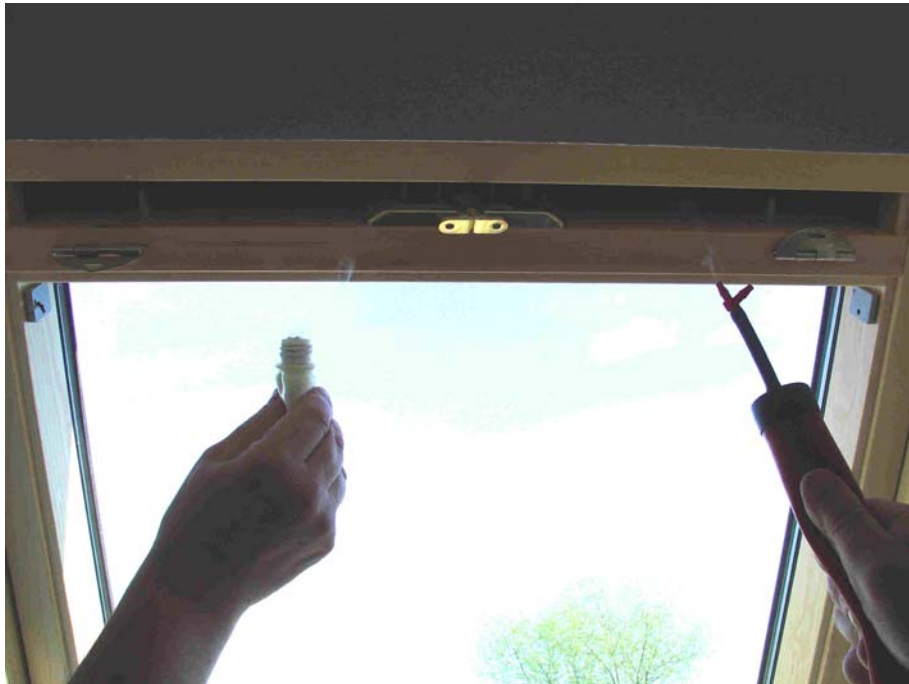
Figure 26 - Leak through Missing Velux Trickle Vent/Handle (Plot 17)
