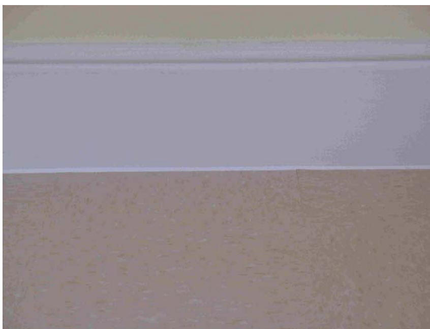
Figure 29 - Sealant used between Skirting and Floor in Kitchen of Unit 4
