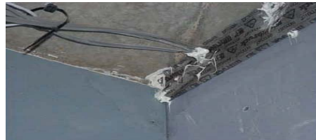
Leakage where membrane is poorly sealed around cables—use of grommets was recommended
