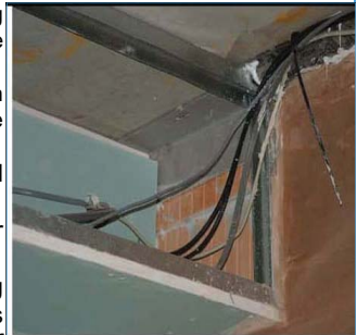
Leakage where section of external wall within services boxing remains unplastered.
