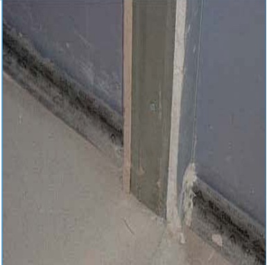
Crack leakage beneath bottom of door frame where membrane seal along base of plaster board is discontinuous.
