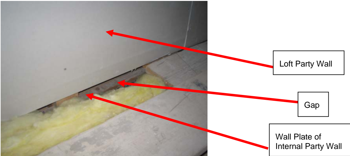
Figure 8 – Gap between Top of Internal Party Wall and Party Wall in Loft
