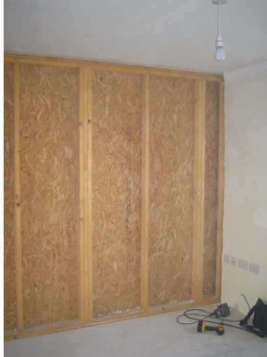
Figure 13 – Exposed OSB Sheathing and Timber Studwork in Party Wall (Living Room No.16)
