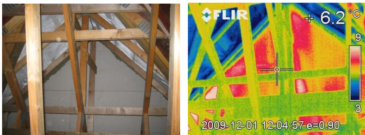
Figure 28 – Photograph and Thermal Image of Party Wall in Loft of House No.15
