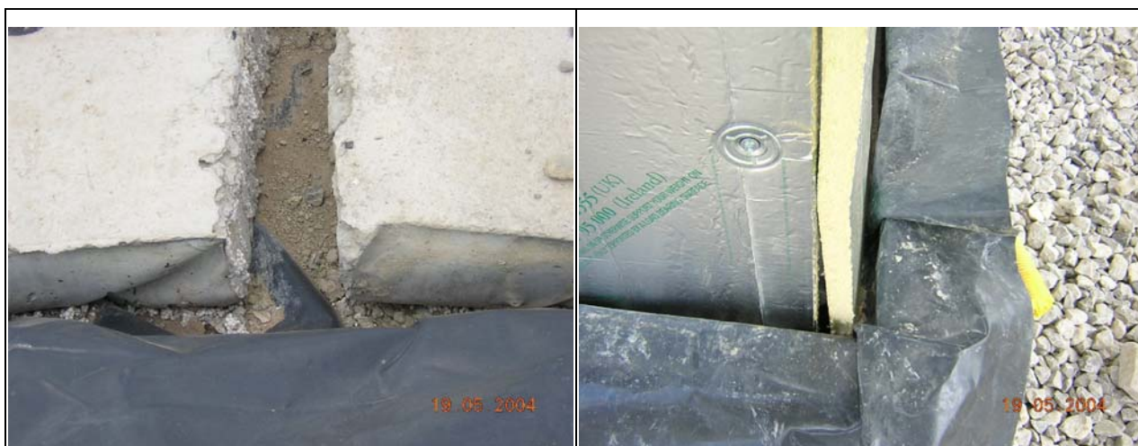
Figure 17 Developer D, Phase 1, the use of removable polystyrene formers created an inconsistent and uneven slab edge, with potential for air leakage at the junction of slab, steel frame and insulation.
