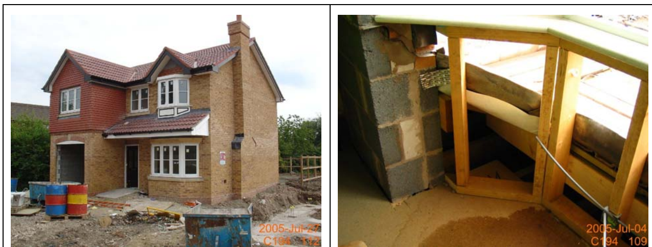
Figure 11 Developer C’s detached property, C194, and internal view of partially constructed first floor bay.
